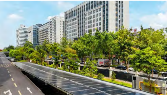
PV Installation on the Company's Parking Canopy Roof
