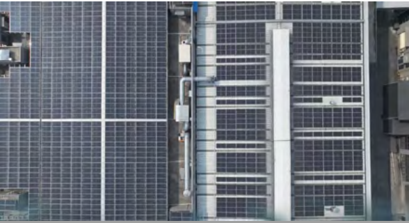
Rooftop PV System
